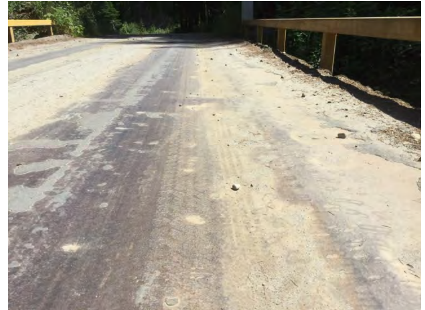
Deck deformation on wheel path
